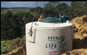
Water and Septic Tanks
